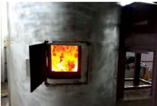
▲ Waste treatment incinerator
