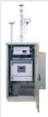
▲ ENVIRONNEMENT S.A air quality monitoring system
